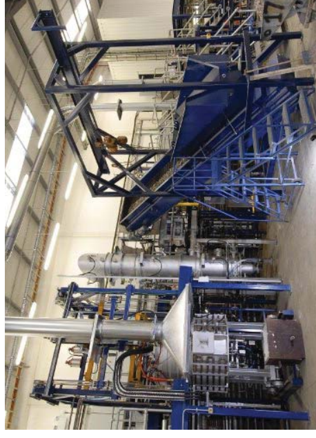
FIGURE 90: GASPLASMA PLASMA GASIFICATION PLANT, SWINDON, UK (SOURCE: ADVANCED PLASMA POWER)
